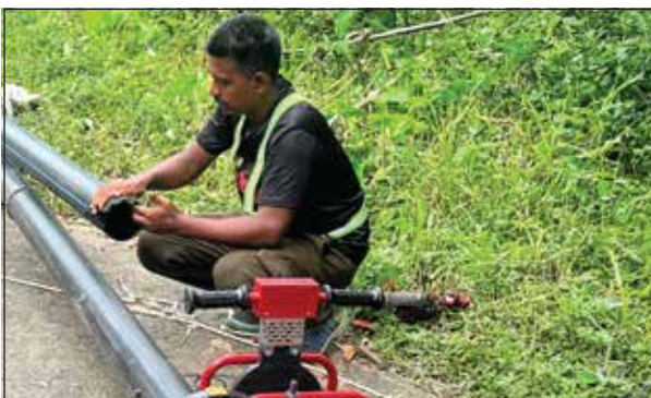
The Purbachall New Town (RAJUK) Project takes trust on RFL HDPE Pipe to transfer Potable water.
